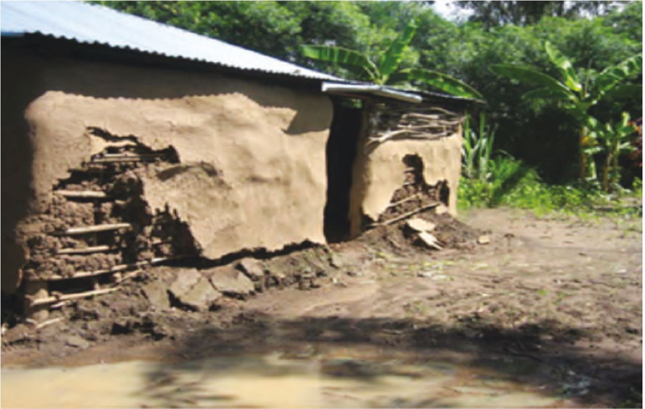
Plate 6.1b: Destruction of houses by floods (a threat to human shelter) in Budalangi, Kenya in 2012 Source: Shisanya (2012)
